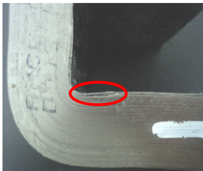
1) Minor gap on top & bottom Surface
